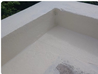
Step 4: Reinforce Neotextile fabric at the base of the wall and the entire floor while the first layer is still wet to increase tear resistance.
