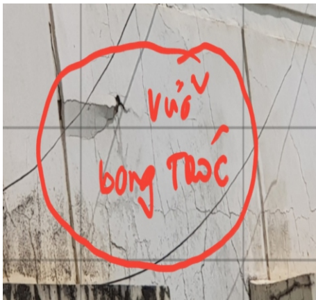
Current Status of peeling surface
