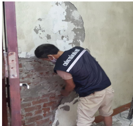
Peel off the peeling render
